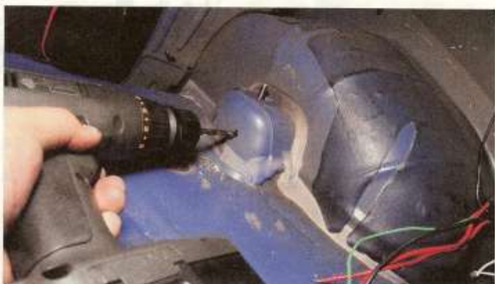
WITH THE panels removed from the truck, we unbolted the shocks and laid the shock lower brace in place to mark the holes. After removing it we were able to drill the required holes to finish the installation.
